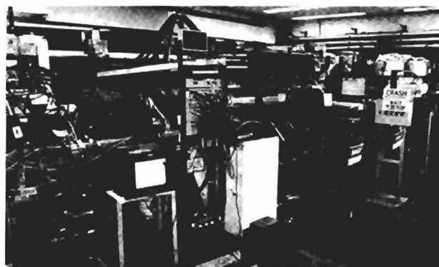
Fig. 6. Bypass interaction range with two of the four BOLD quadrants mounted in place.
