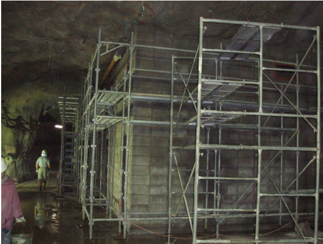
Control room for the distillation system in the newly excavated mine tunnel
