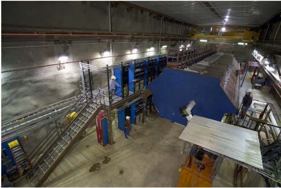
Figure 4.7: The Near Detector fully installed underground at Fermilab.
