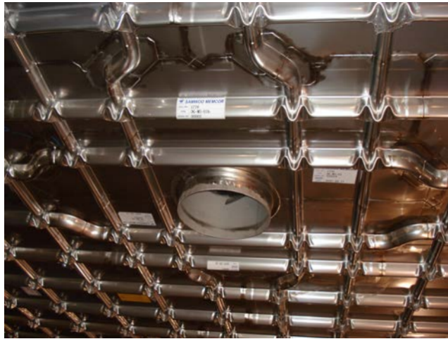
Figure 2.3: Nozzles in the roof of membrane cryostat (Figure courtesy GTT).
