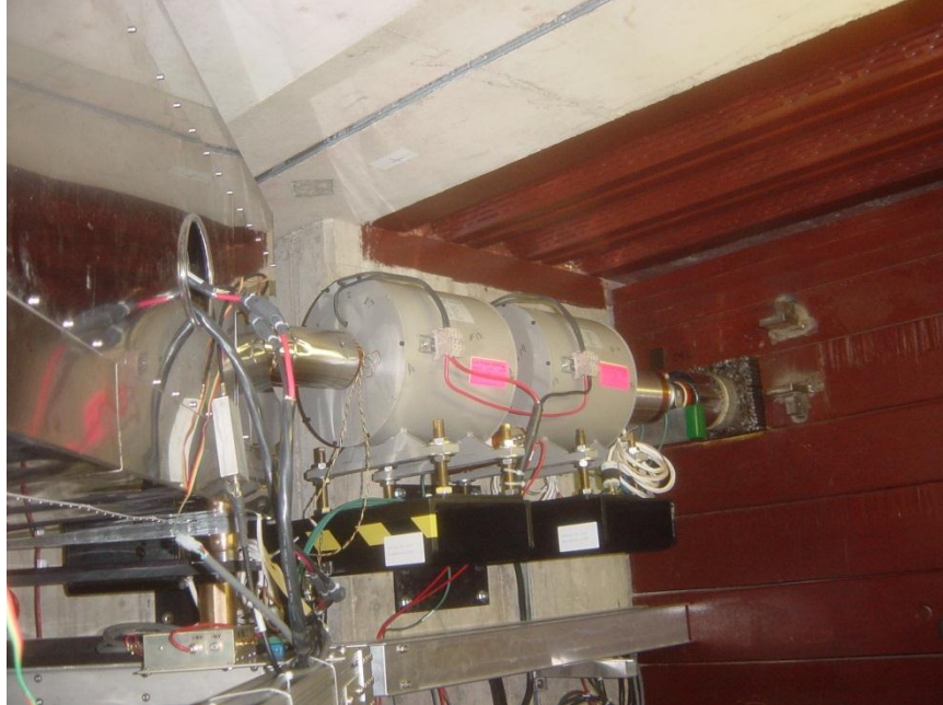
Figure 9. A doublet of solenoidal lenses in the supply line inside the MI tunnel. The red wall on the right is radiation shielding of a line toward the Pelletron. The shiny box on the left is the magnetic shield of the bend that merges the electron and antiproton beams. Parts of the beam line outside of the focusing elements are covered by \mu - metal magnetic shield. The transfer line is below.
