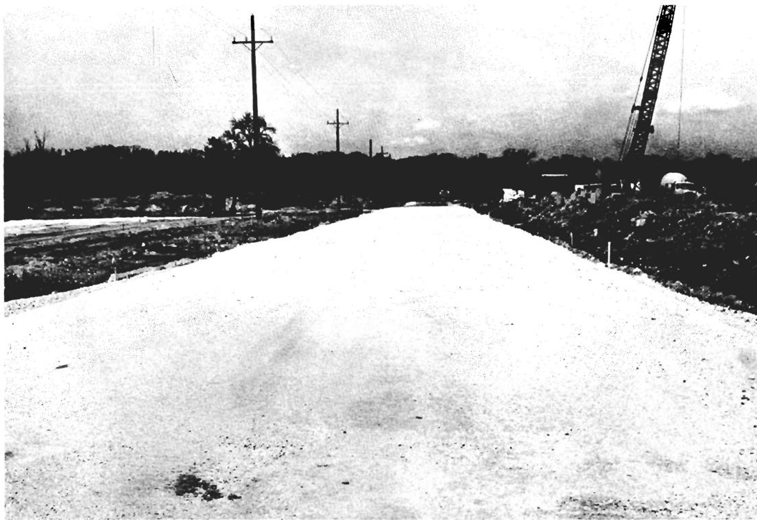
Fig. 4. Progress on the main road. The linac building is to the right.
