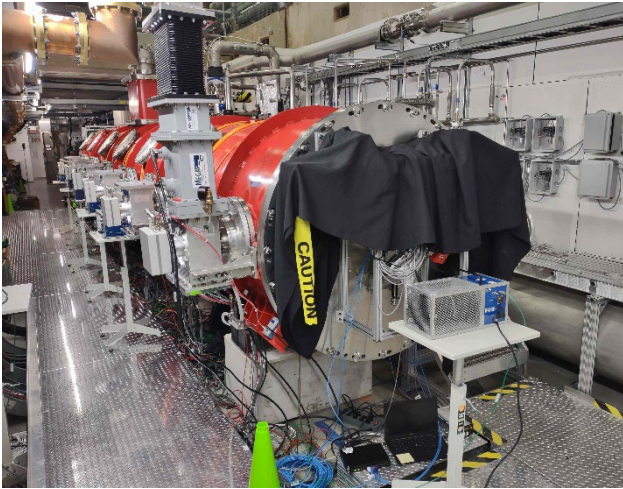
Figure 3: HB650 pCM installed in PIP2IT for post-transport testing at 2K
