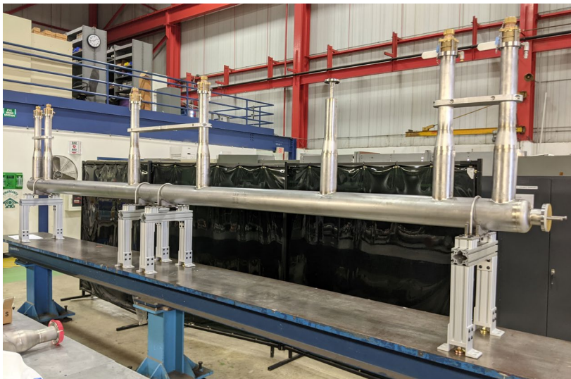
Figure 1. Adapter transfer line used to accommodate HB650 cryomodule U-tubes prior to installation in the PIP2IT cave
