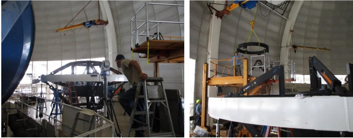
Figure 6: Left-The DESI cage being centered relative to the upper ring on the Mayall C floor. The spider vanes' lengths were adjusted to move and orient the cage, with positioning feedback from the laser tracker in the foreground. Right-The top ring of the cage being lowered onto the yellow Southeast Platform, after temporary removal to allow installation of the corrector and hexapod into the cage.
