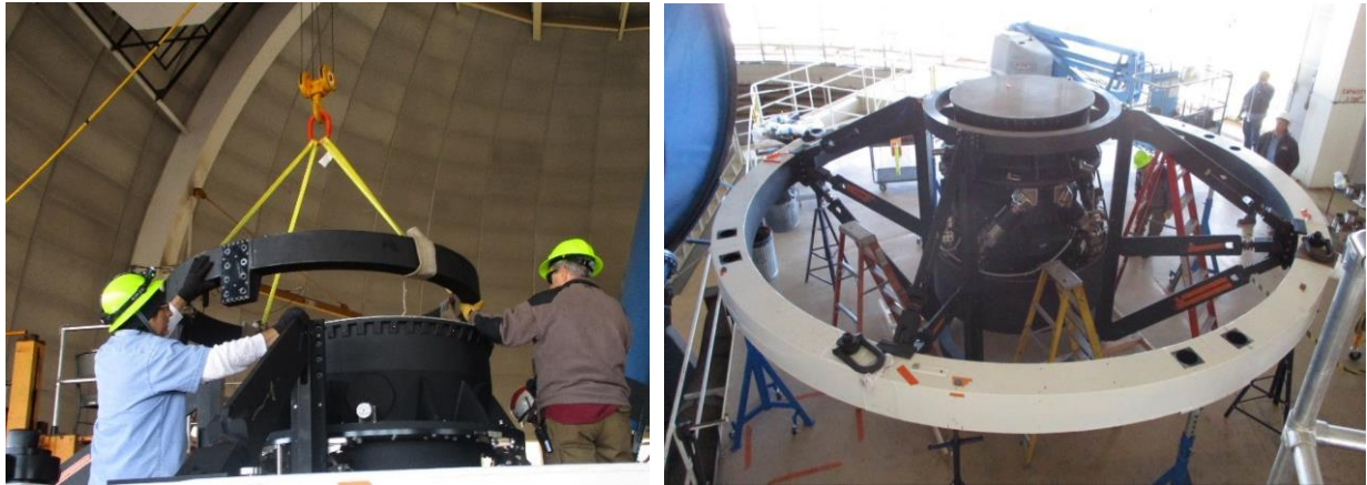
Figure 8: Left-The cage top ring is reinstalled after the corrector and hexapod installation to the cage. Right-The corrector/hexapod installed in the cage, with the cage upper ring reinstalled, the corrector centered relative to the upper ring, and the vanes adjusted to their in-service tensions.
