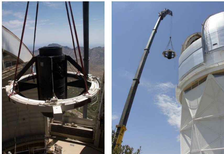
Figure 2: Left-The old Mayall prime focus cage, support vanes, and support rings being lifted away from the telescope through the open dome slit. Visible through the dome slit are part of the crane boom, the nearby Coyote Mountains, and the
