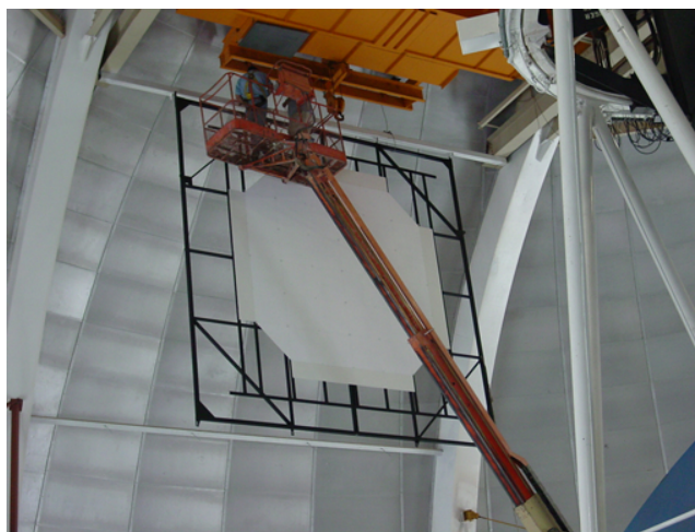
Figure 8.4: Installing the existing reflection screen used for daytime flat fielding. The screen is being mounted to the inside of the dome, between the arch girders and just below the attachment point for the dome crane rails. Note the use of a long-reach boomlift. For safety reasons, the telescope drives must be locked out and tagged out during the entire operation.
