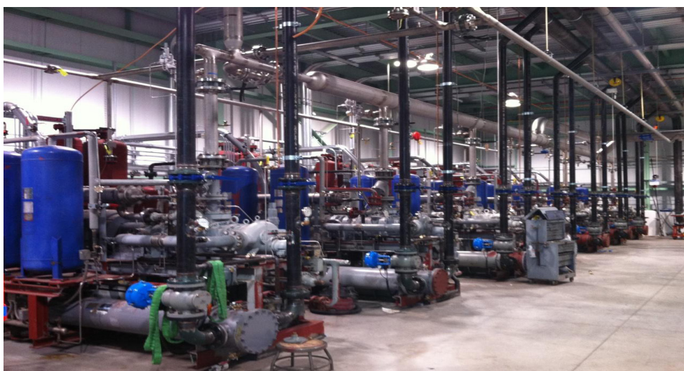
Figure 2. CMTF Warm Compressor Room
