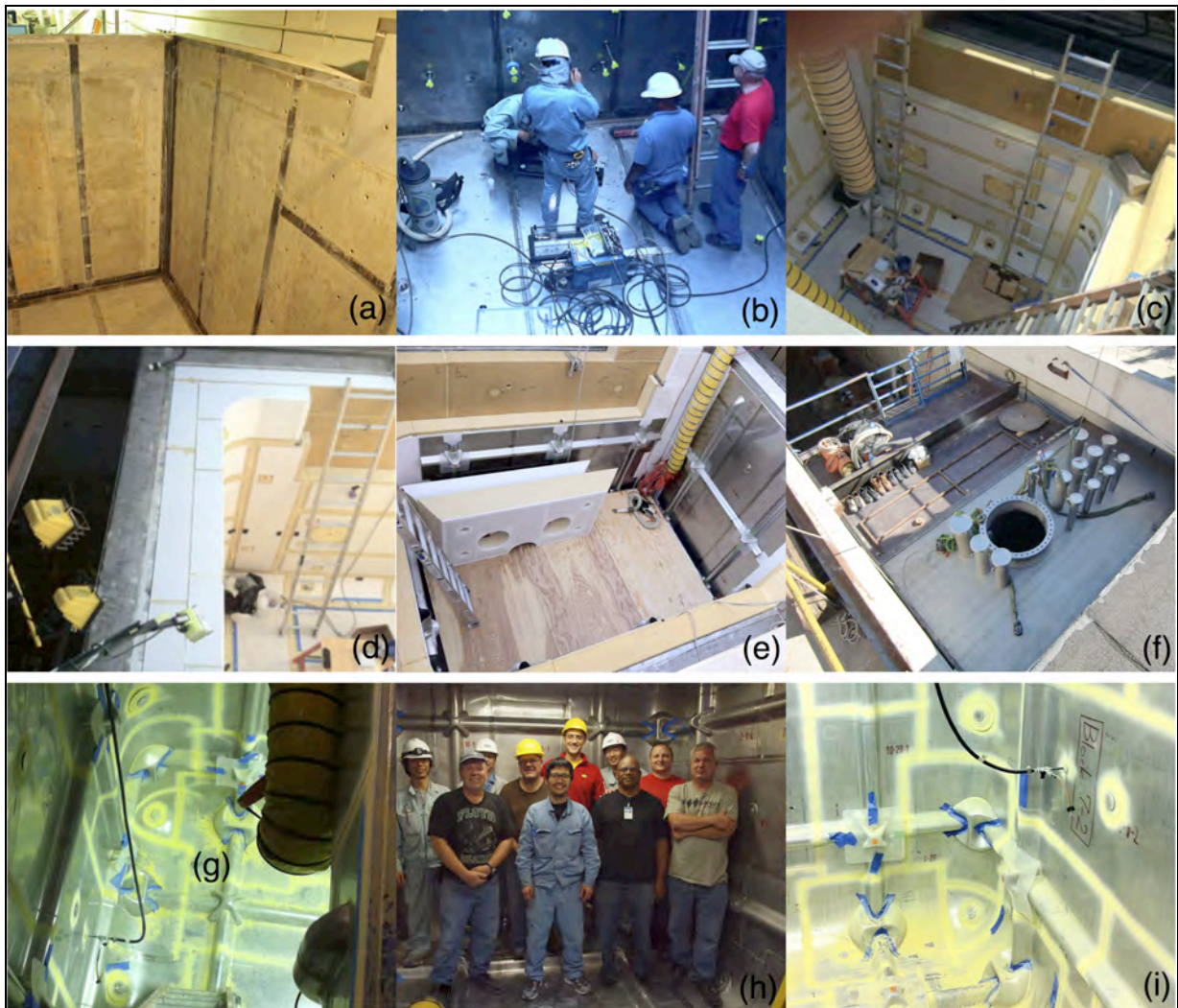
FIGURE 4. Photos during construction: (a) Concrete structure before starting the installation of the vapor barrier; (b) Test of the vapor barrier with vacuum box; (c) Installation of the inner layer of insulation; (d) Top view during the installation of the second layer of insulation; (e) Installation of the membrane; (f) Top view of the completed membrane cryostat; (g) Ammonia leak check of the membrane cryostat; (h) Partial group photo after the completion of the installation, and (i) Ammonia leak check of the membrane cryostat.
