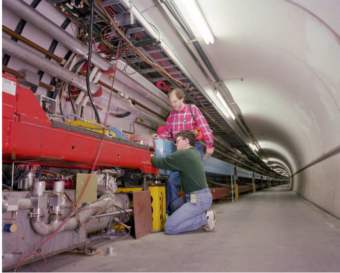
Figure 1. View inside the Tevatron tunnel. Image courtesy of Fermilab Visual Media Services.
