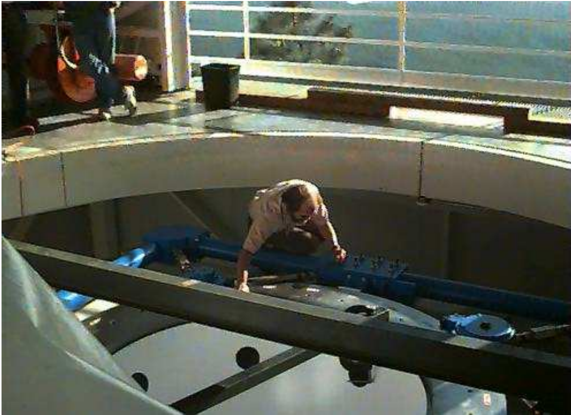
Fig. 25.— The azimuth support is installed and tested. This image shows the inspection of the azimuth drive disk.
