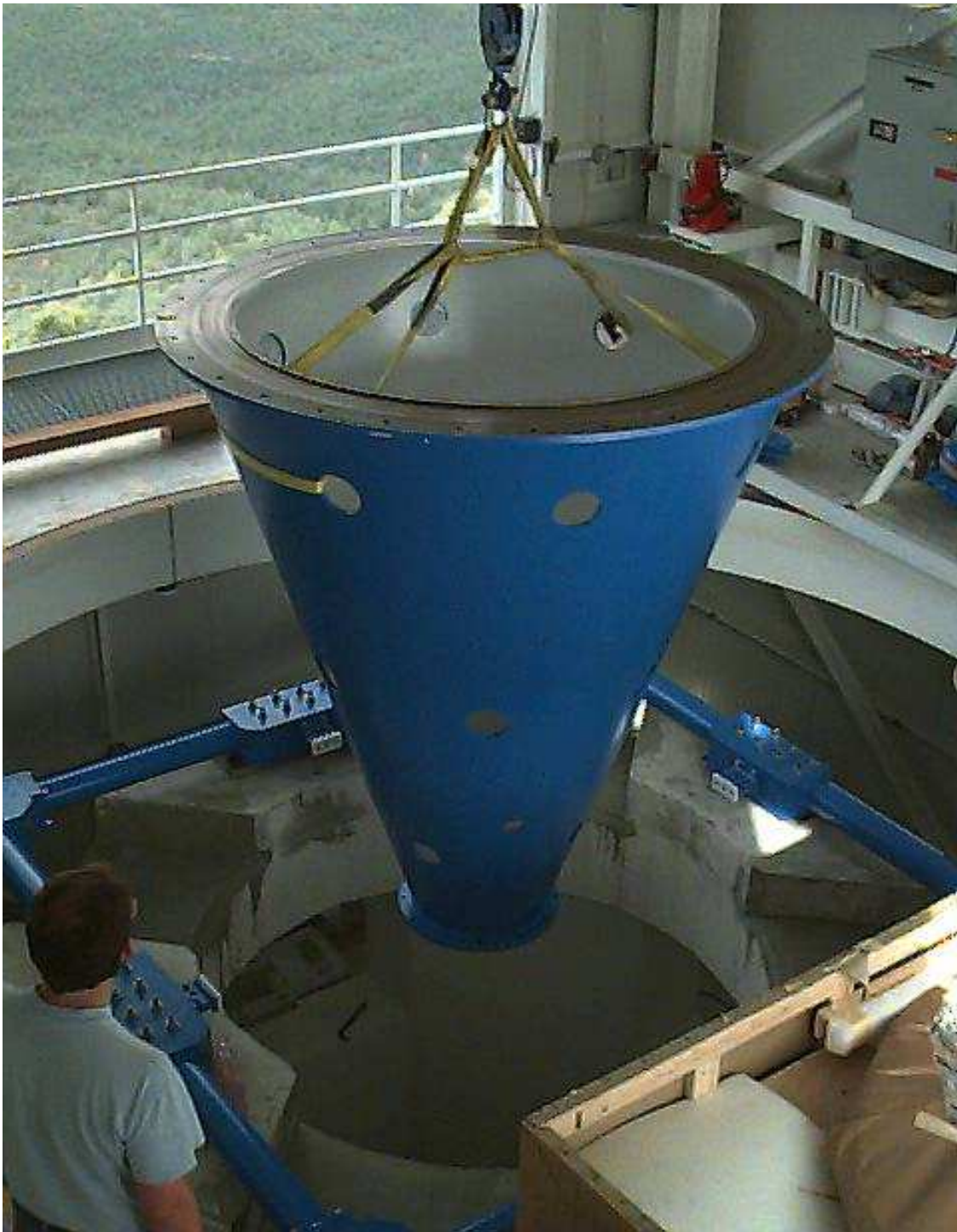
Fig. 24.— Installation of the SDSS 2.5 m telescope begins in earnest. On August 15 1995 the azimuth bearing and support is lowered into place through the floor of the support platform (see Figure 12).
