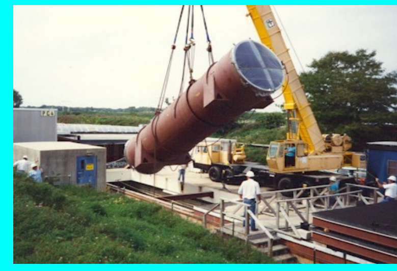
The SELEX RICH detector vessel being installed in the MIPP hall, before the hall was enclosed.
