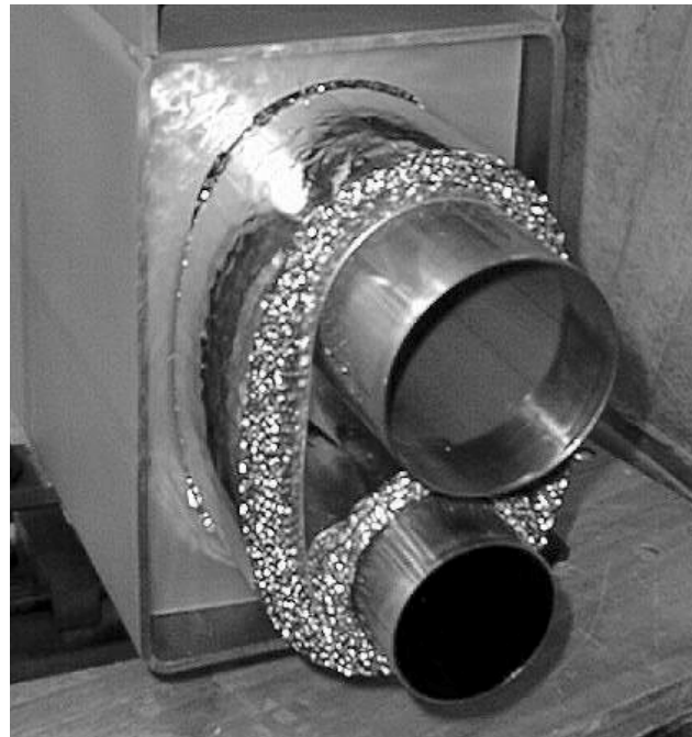
Fig. 17 – Photograph of the cryogenic supply and return lines of the 2m prototype. Dimpled aluminized Mylar is wrapped around the 2-pipe package as well as the smaller 3" supply line.
