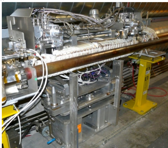
Figure 5-3: Photograph of the active absorber TCLA.B6R7.B1 as installed in the betatron cleaning insertion.
