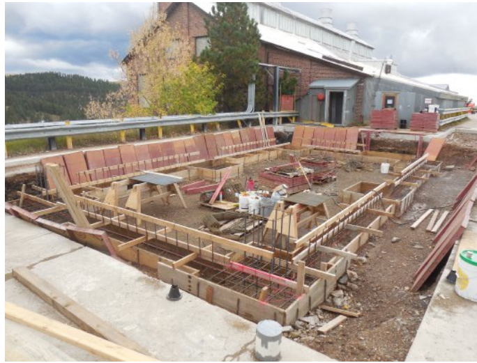
Figure 10.1.3: A picture (October 2016) of the additional building being constructed to house the radon-removal system (RRS).
