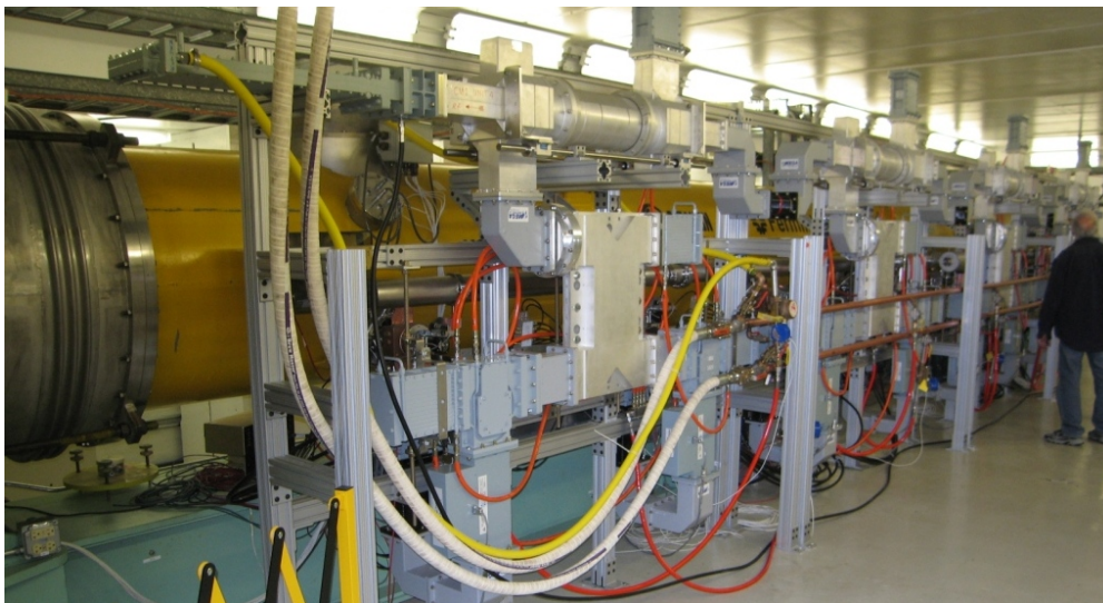
Figure 6: Photograph of cryomodule I installed in the ASTA beamline enclosure. View is looking downstream. Waveguide distribution structure is on the right of the cryomodule.
