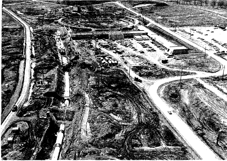
Fig. 2. Progress of work on the main ring. The Transfer Hall and Injection Area are in the distance. Road A is at the right and the Ring Road at the left. The excavation for the first Vehicle Access is at the far end of the Transfer Hall. The excavation inside the ring just this side of the two utility poles is the beginning of the first service building.
