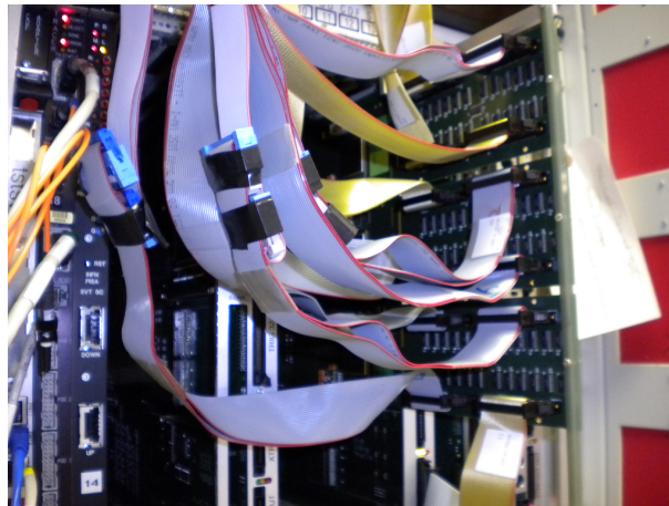
Figure 4.7: The GigaFitter system in the test crate of SVT. All 12 inputs are connected in parasitic mode to split HB++ outputs.
