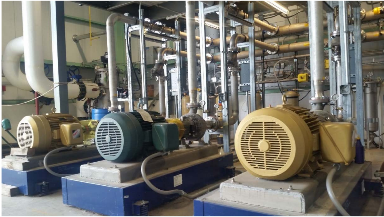
Figure 4.6: Typical LCW pump room.
