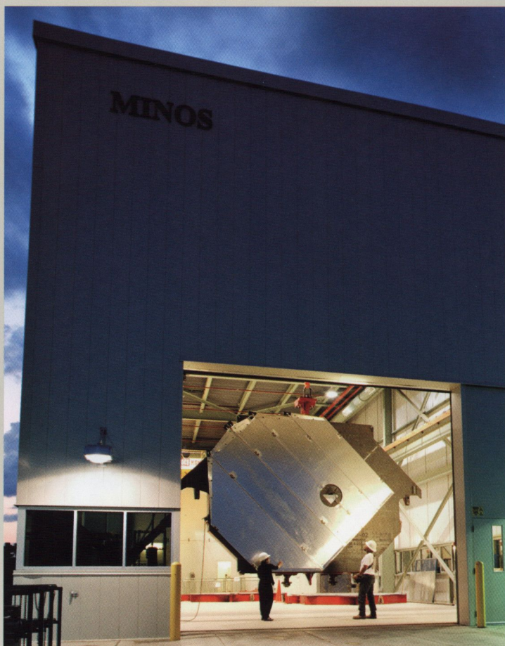
Workers move a detector plane of the MINOS neutrino experiment into place to lower it underground for installation in the MINOS near detector. (Photo credit Peter Ginter)
