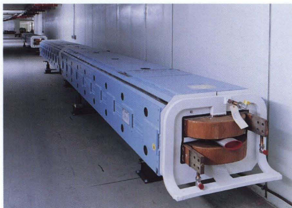
New magnets in the Main Injector tunnel.
