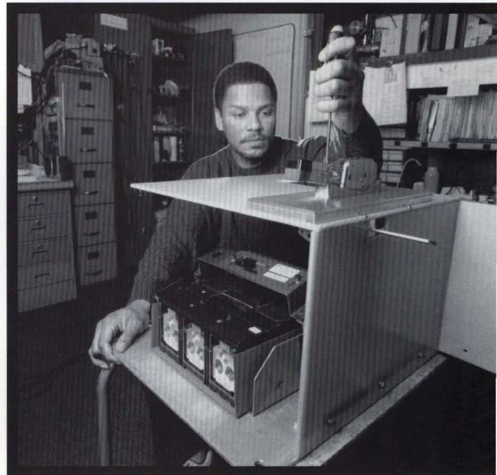
A member of the Accelerator Division's Electrical and Electronics Support Group, Leroy Middlebrooks adjusts the control mechanism on a safety switch assembly for a power supply. This switch provides technicians a safe means to disconnect and to lock off the incoming 480-volt, three phase power. The group designs, builds and tests the specialized electrical equipment required by the division, and in 1992 was heavily involved in the low-beta project and the Linac upgrade.
