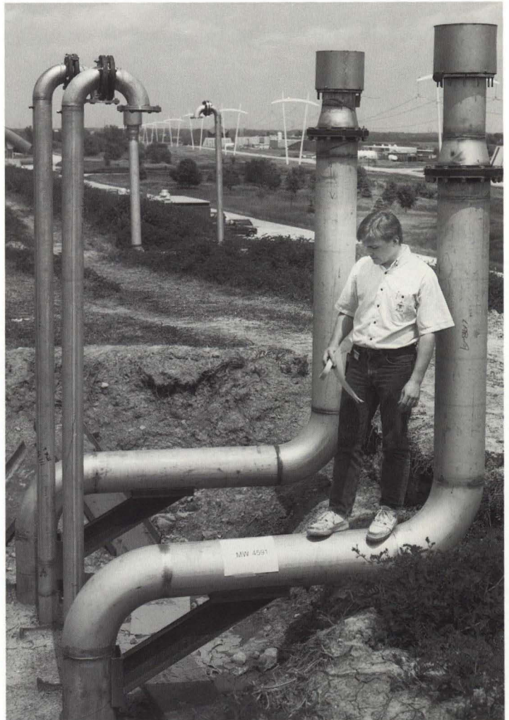
Bruce Squires examines the reinstallation of the cryogenic relief valves on the Meson berm. During the 1991 shielding project, the valves, which vent gaseous helium and nitrogen in the event of a magnet quench, were heightened and offset in order to reduce radiation danger in the event of an accident in the beam directly below.
