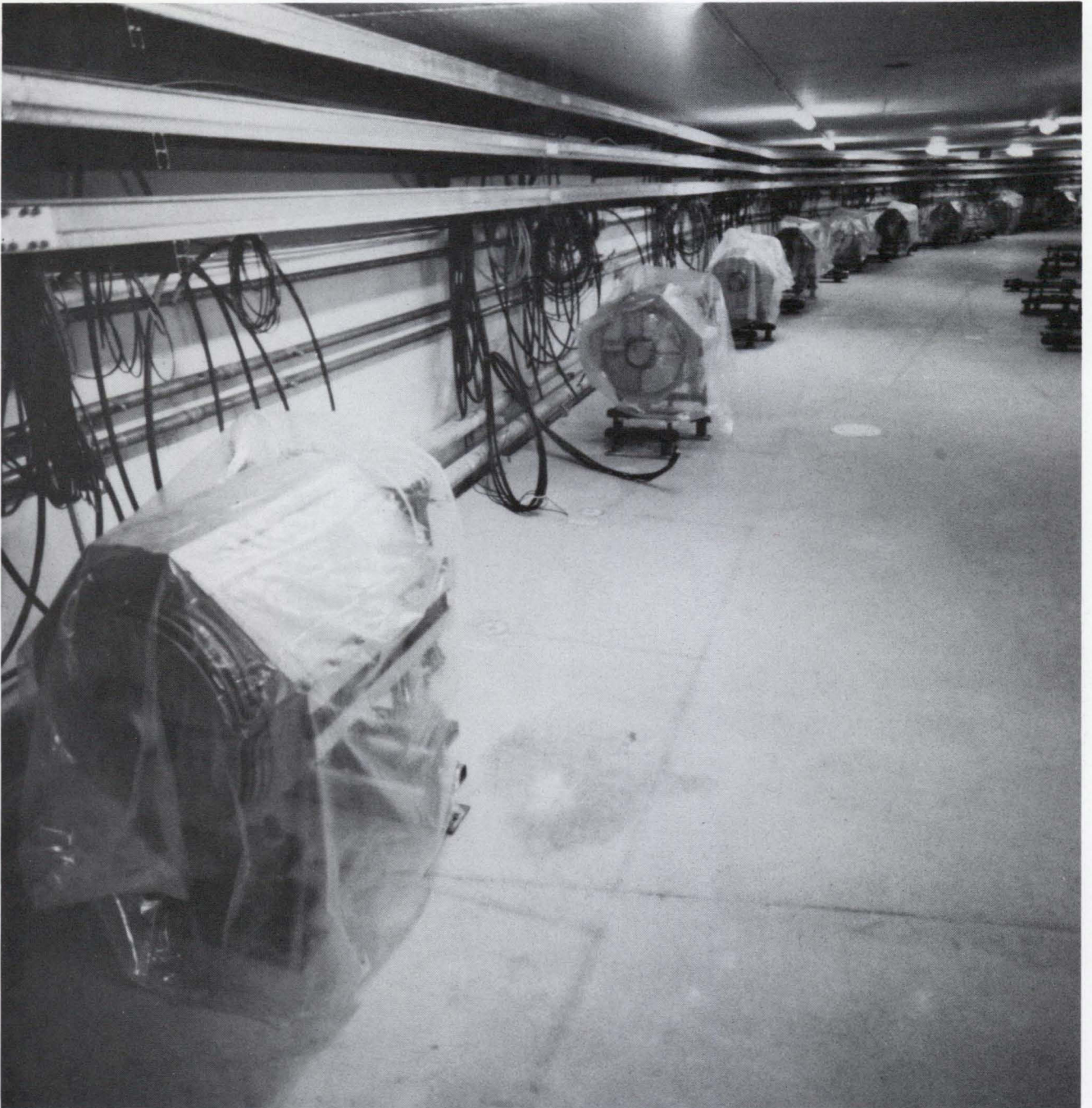
Debuncher quadrupoles installed in the tunnel.
