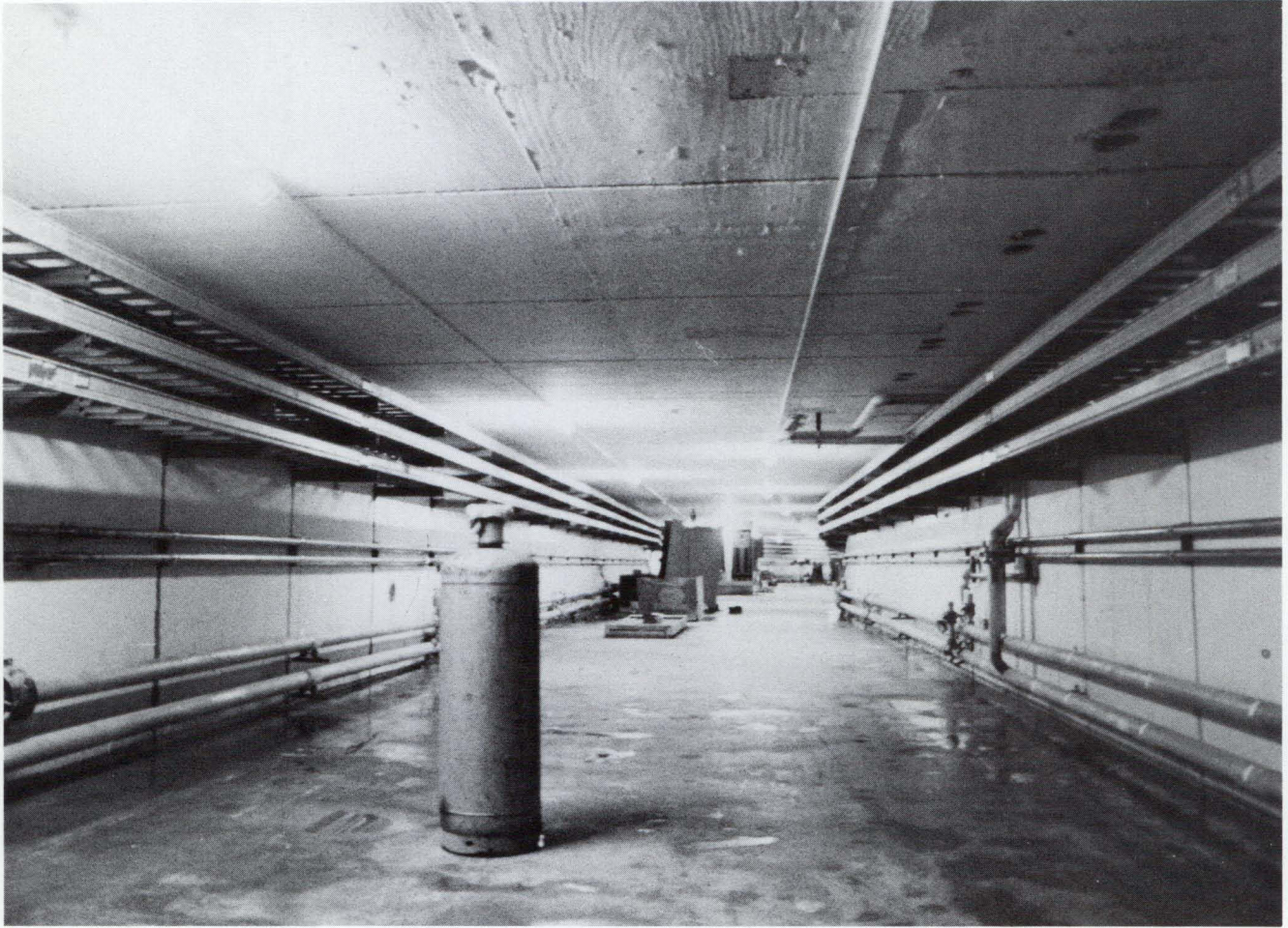
The Antiproton Source tunnel, prior to installation activities.
