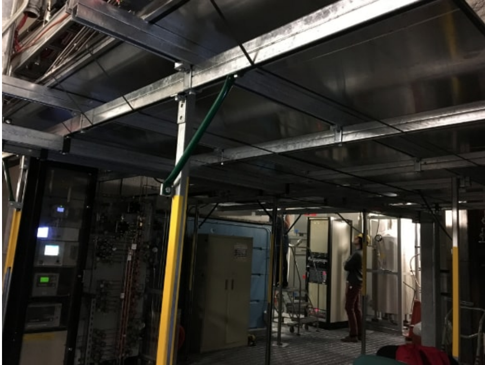
Figure 13: MicroBooNE CRT showing the bottom plane and its support structure
