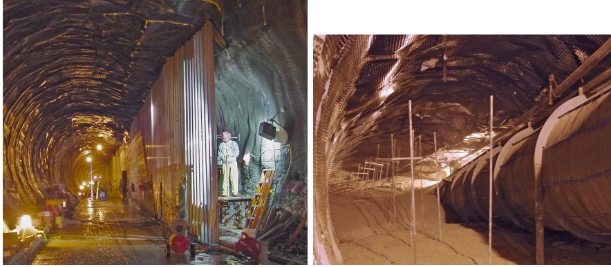
Figure 17: The NuMI Decay Pipe Tunnel. The left photograph shows the decay tunnel before the decay pipe was installed. The wall was the form for the concrete shielding and the worker shown was standing in the egress passage. The right photograph shows the installed decay pipe with concrete shielding being poured. The stiffening ribs around the pipe are also visible as well as the copper cooling lines running along the length of the pipe.
