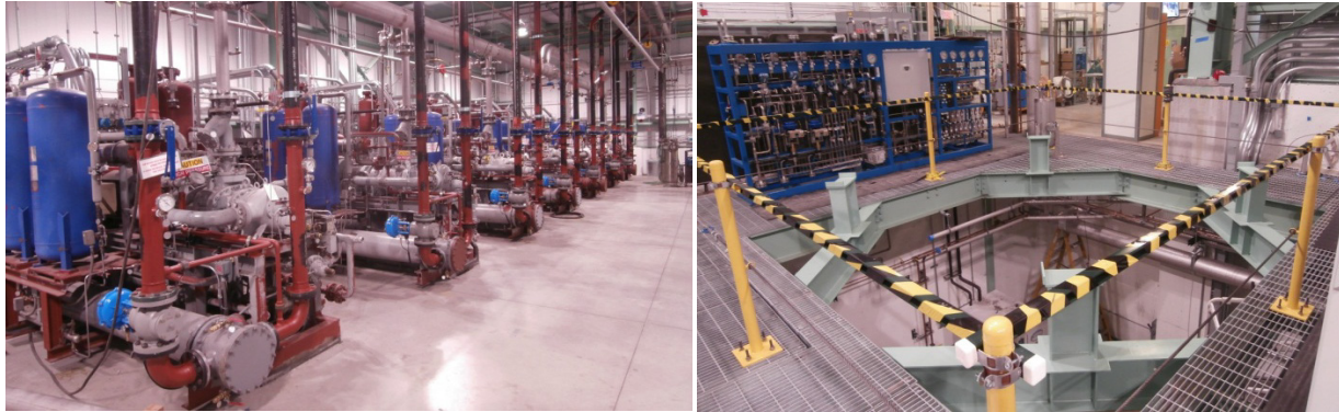
FIGURE 3. Photograph of the CMTF Compressor Room (left) and the SCP Pit and Instrument Panel (right)
