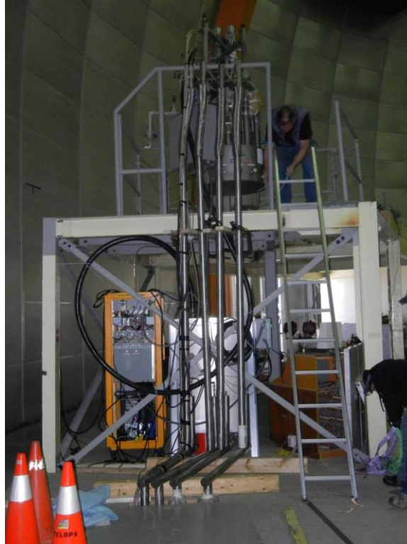
Figure 3. LN2 process station mounted to top of old console room roof. In the old console area is the slow controls rack. LN2 transfer lines are routed from the LN2 process station to the Coudè room and to the Telescope.
