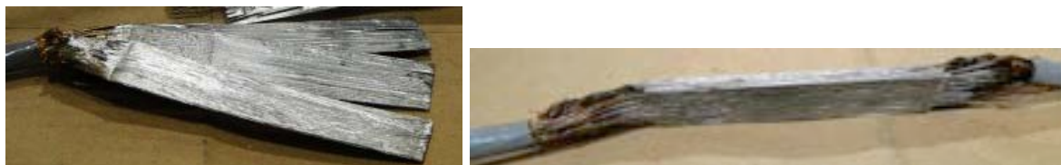
FIGURE 7. Practice sample of 13 kA bus tinned for final soldering (left). Practice sample of 13 kA bus cables soldered together (right).
