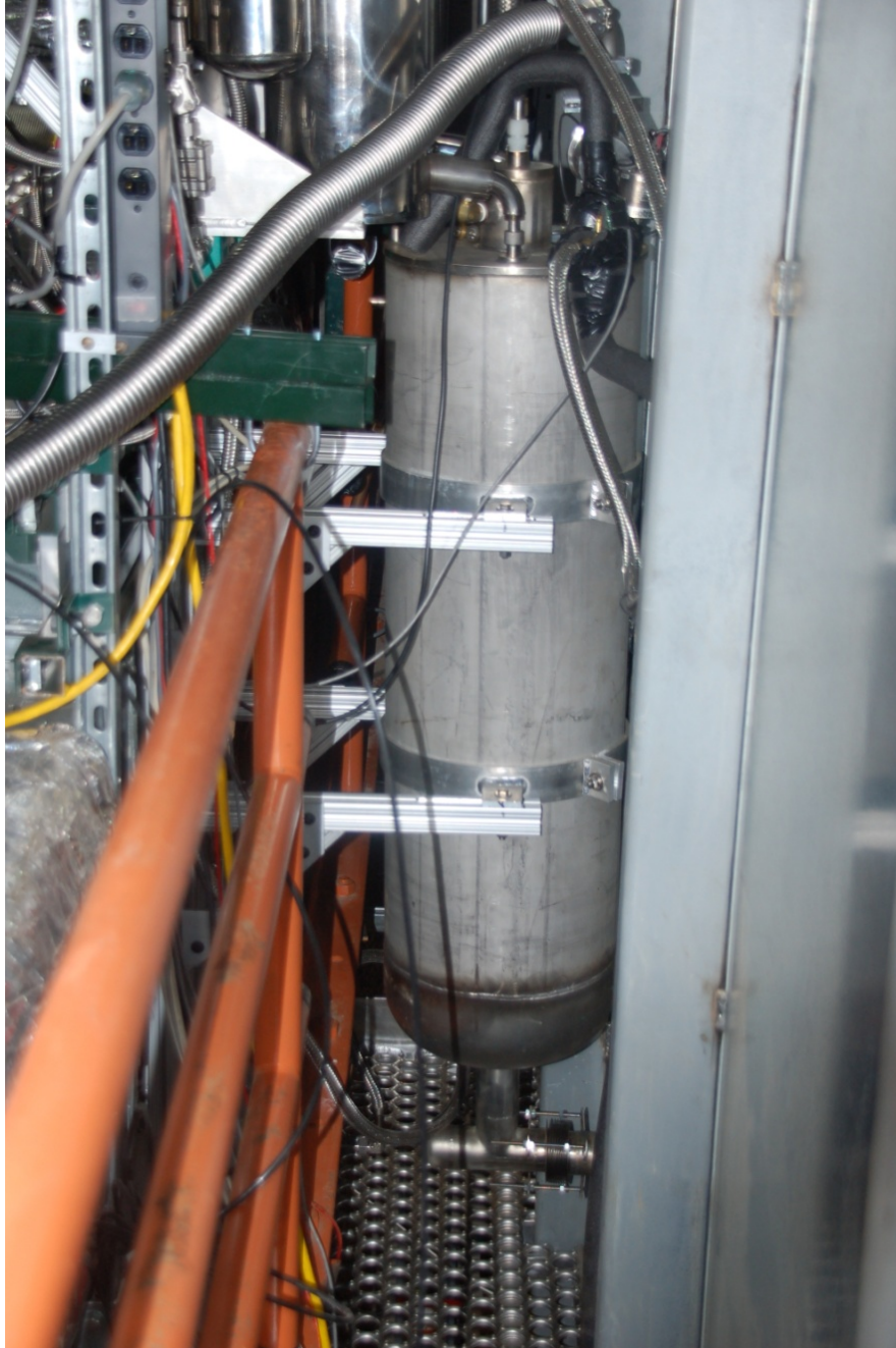
FIGURE 4. Transfer line outside the RF room showing re-liquefier drain leg, nitrogen connections and bottom connection through the RF room wall on the right
