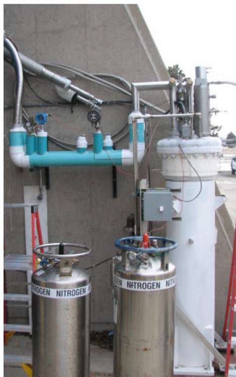
Figure 1. Liquid nitrogen vessel and foam insulated valve box located outside the building.
