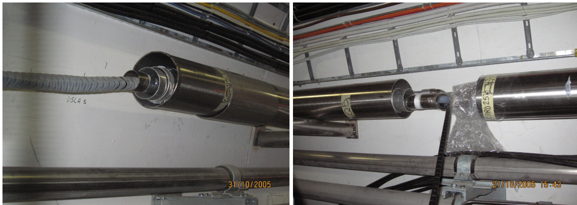
FIGURE 6. Cable bundle insertion in type-1 DSL (left), and extraction at a branch (right).
