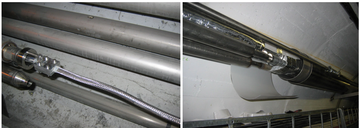
FIGURE 7. Type-2 DSL view of cable with wavy over-length pattern and clamp (left), general view of DSL at thermal compensation location (right)
