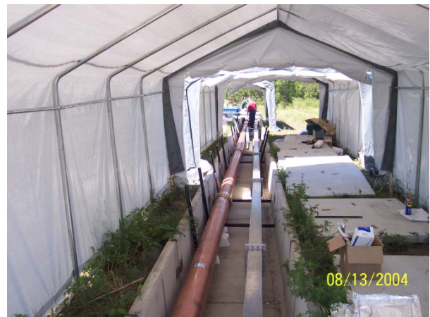
Figure 8: Picture of the high power 805 MHz and 201 MHz transmission lines at top of linac shielding being installed to the MTA.
