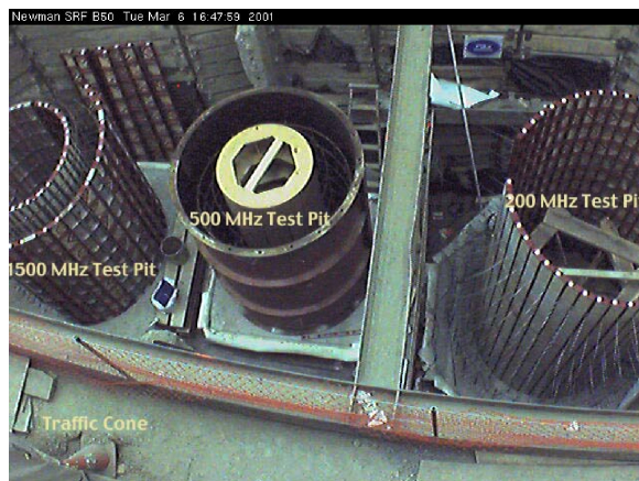
Figure 14.10: 200 MHz test pit (2.5 m diameter and 5 m deep) under construction at Cornell. The other pits are for testing existing cavities.
